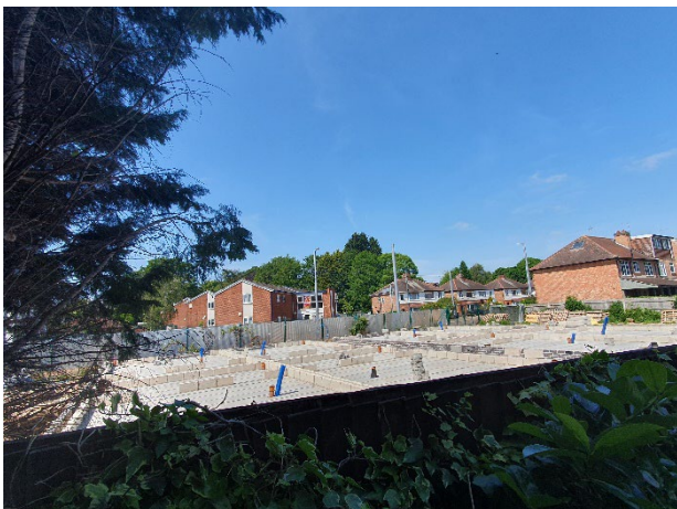
Wider site, permission being constructed under 21/01055/FUL – facing north west from rear footpath
